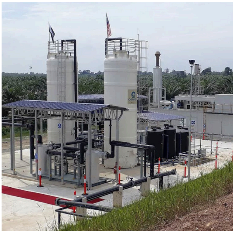
Plant: Sri Jelutung Palm Oil Mill, Malaysia. Capacity: 800 M3/h (470 scfm) biogas 3,000 ppm H2S
