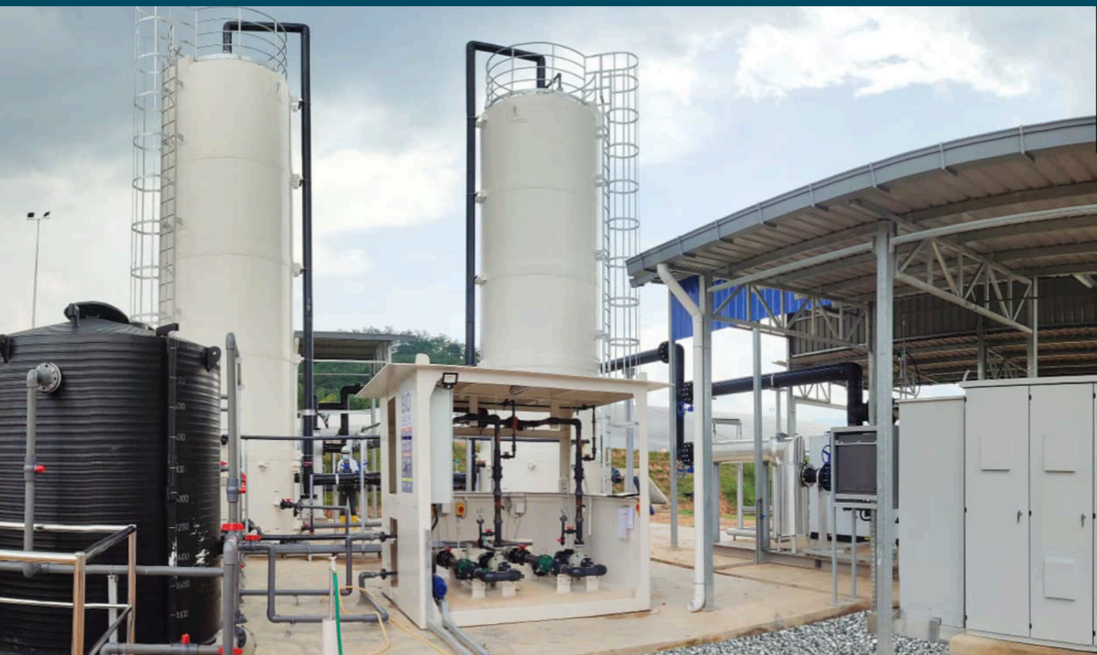
Plant: Elphil Palm Oil Mill, Malaysia. Capacity: 800 M3/h (470 scfm) biogas 3,000 ppm H 2 S
